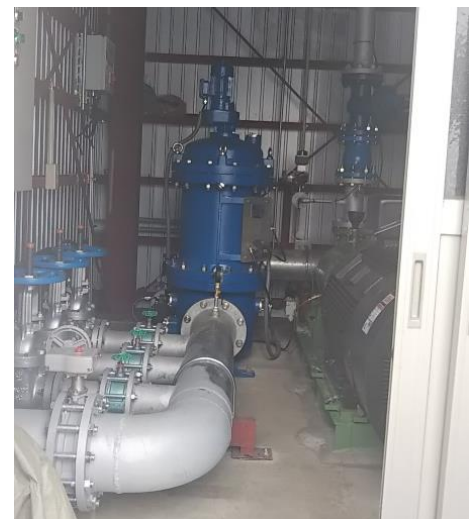
Filter system in the pump station
