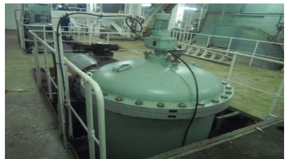
Picture 3: BOLLFILTER Automatic Type 6.18.3 installed
